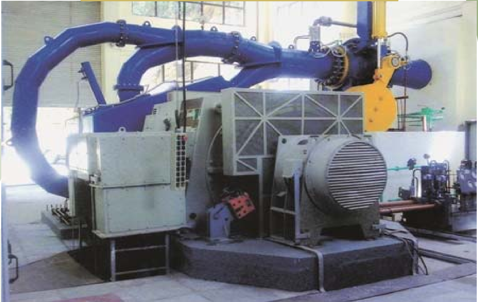
4.5 MW Capacity SHP Generator at Manglad, Himachal Pradesh
